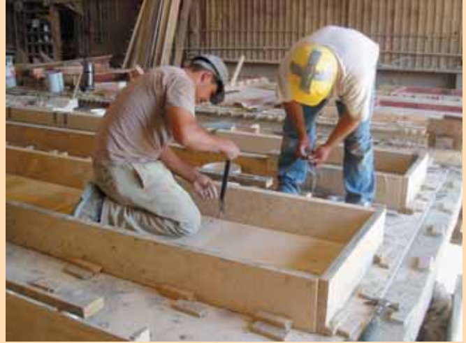
Precasting the concrete panels for the building’s bands called for precise work; the tolerance of \pm \frac{1}{64} " is twice as small as what’s often used. (Photo courtesy Enterprise Precast)
